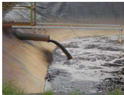
Landfill leachate entering retention ponds for treatment.
